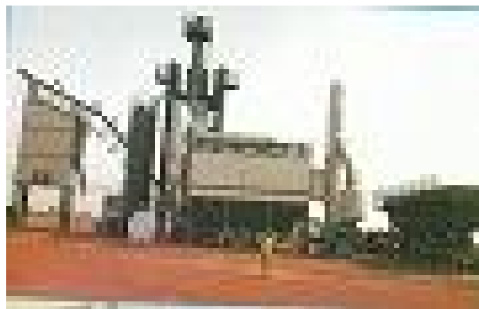
One of the re-activated Asphalt Plant in the State.
