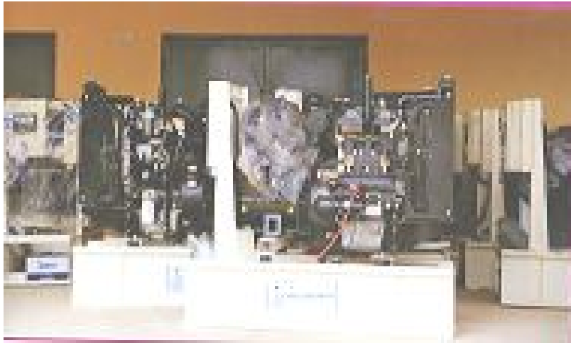
Some of the generators supplied by Gov. Geidam's administration
